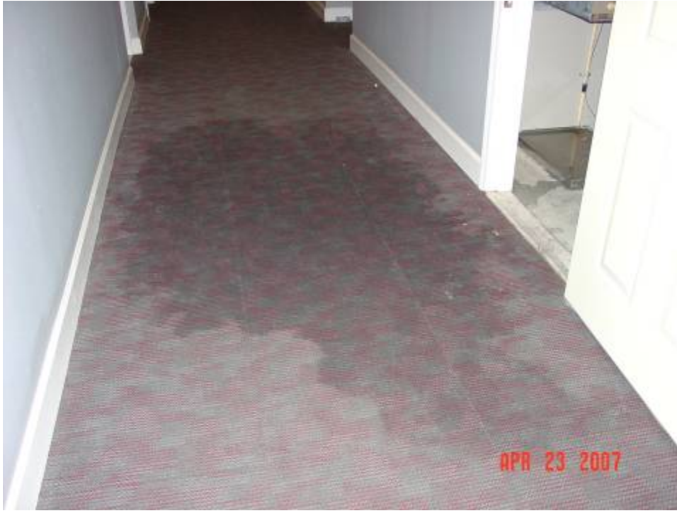
Water damage to hallway from overflowing condensate drain pan.
