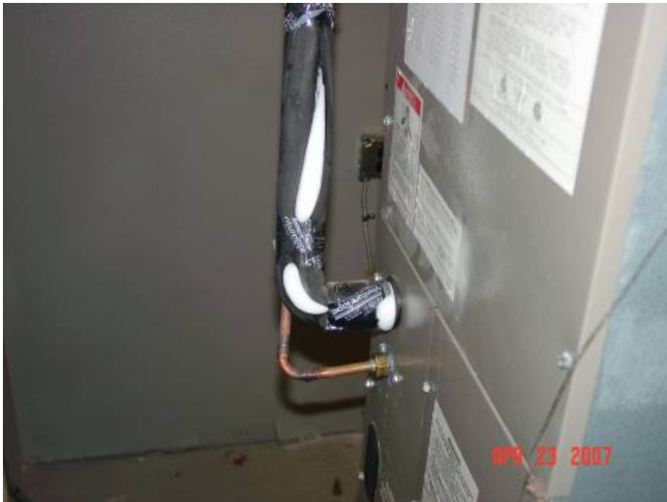
Frozen suction line at air handling unit.
