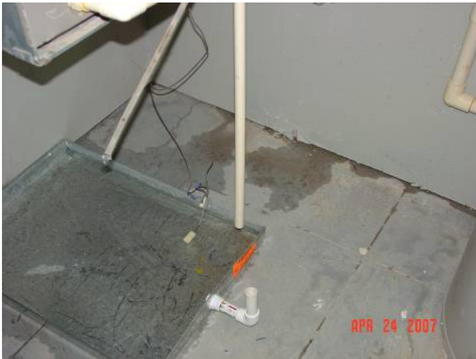
Condensate overflow into wall cavity.
