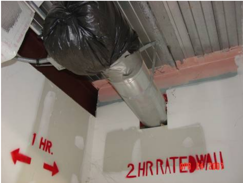
Fire-rated wall not properly sealed.
