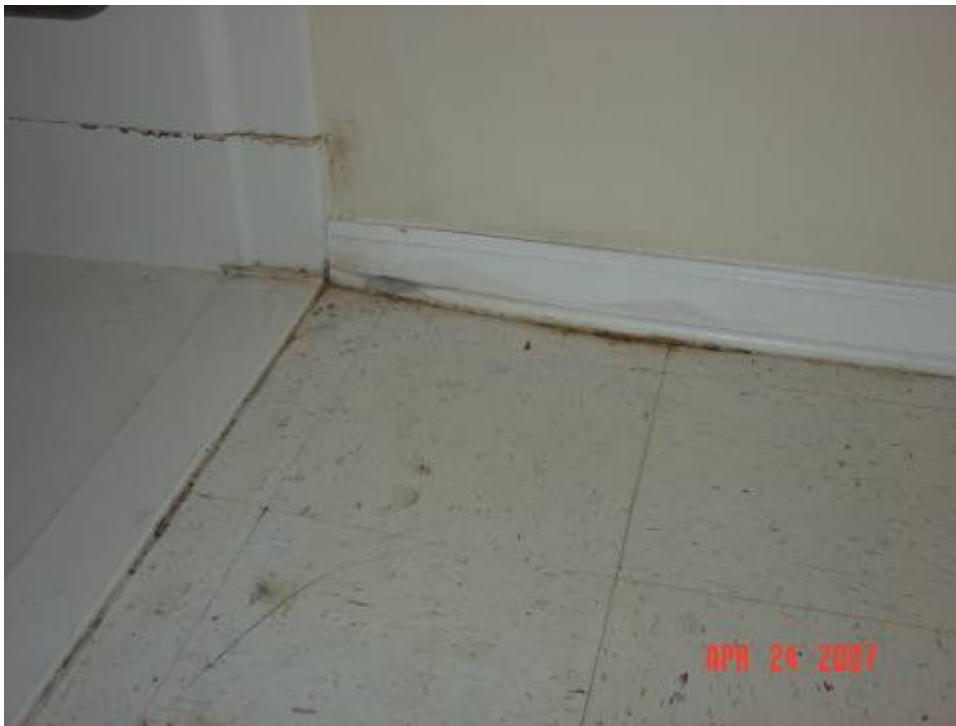
Moisture damage from shower.
