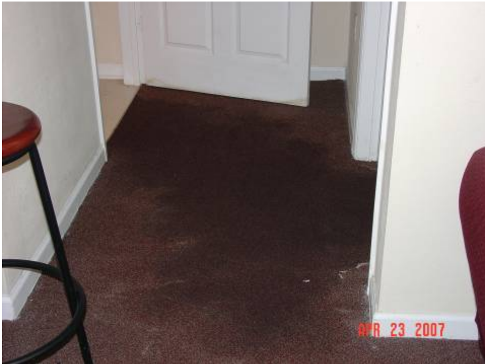
Water damage in student suite from plumbing leak.
