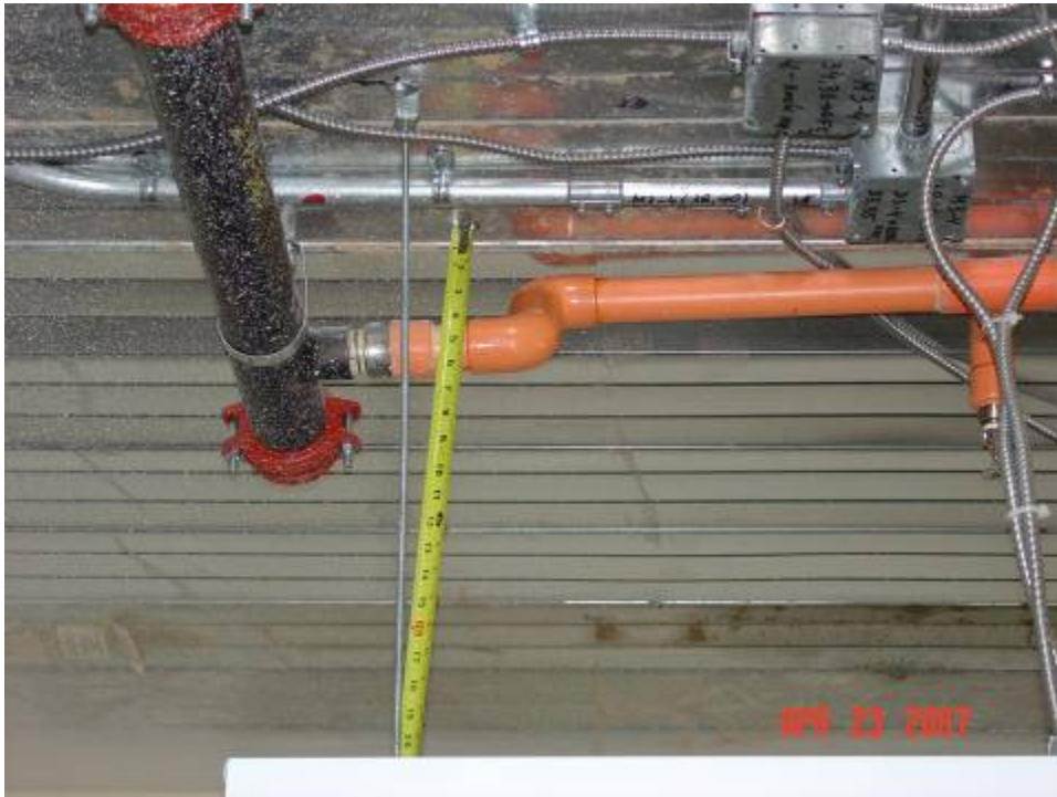
Plastic sprinkler pipe not routed flush to ceiling.
