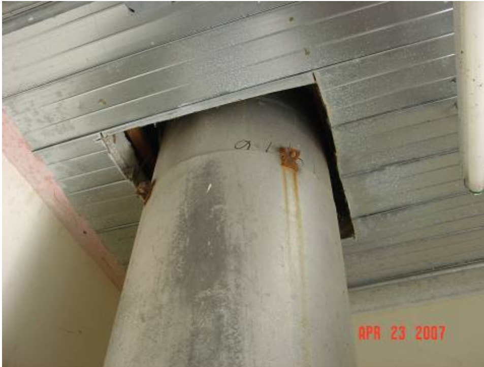
Bottom of trash chute chase not sealed.
