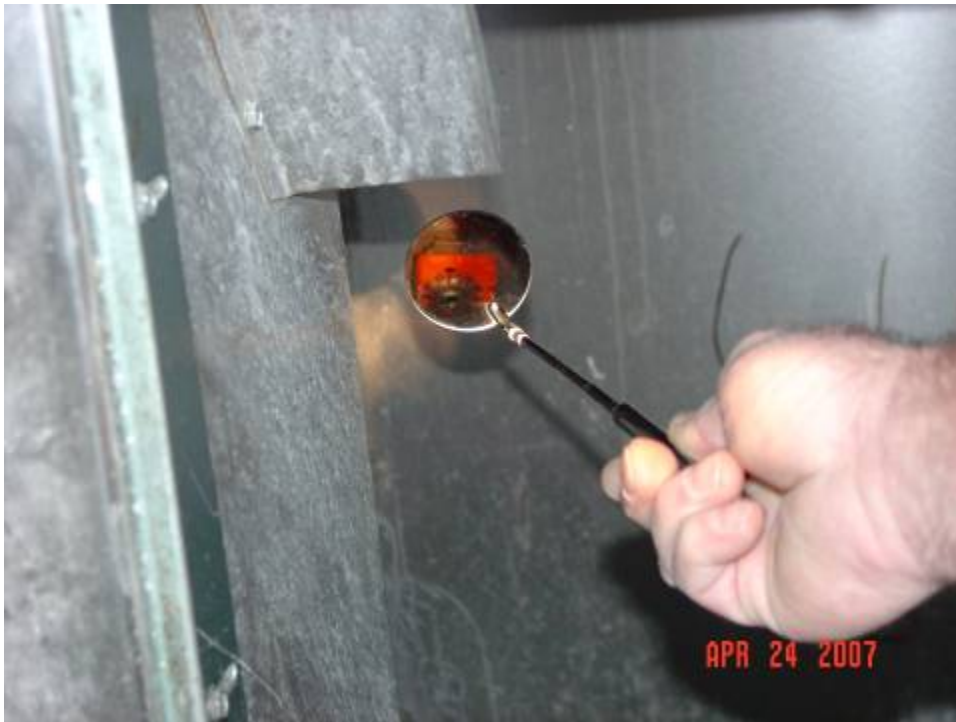
Plastic tab covering sprinkler head fusible link.
