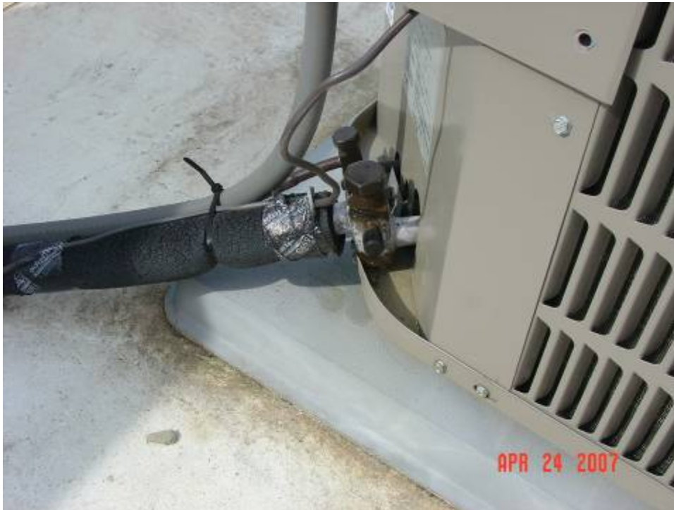
Frozen suction line on heat pump.
